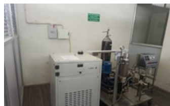
Super Critical Fluid Extraction Unit
